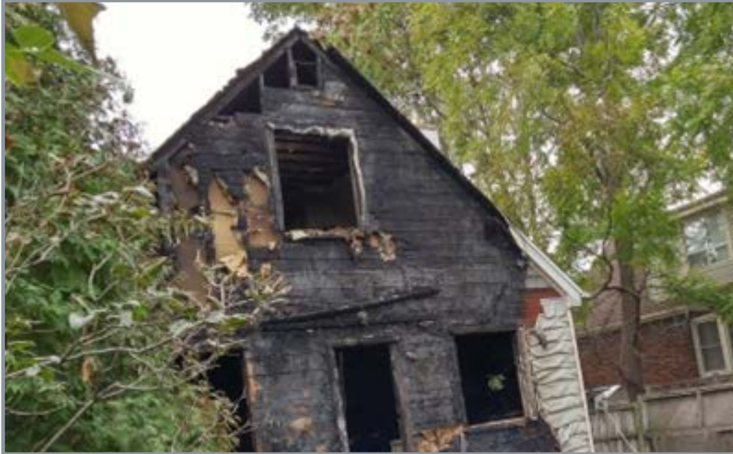
Fig. 3: 2016 Hamilton house fire killed 3 in house improperly zoned as a single-family home (CBC). 19
